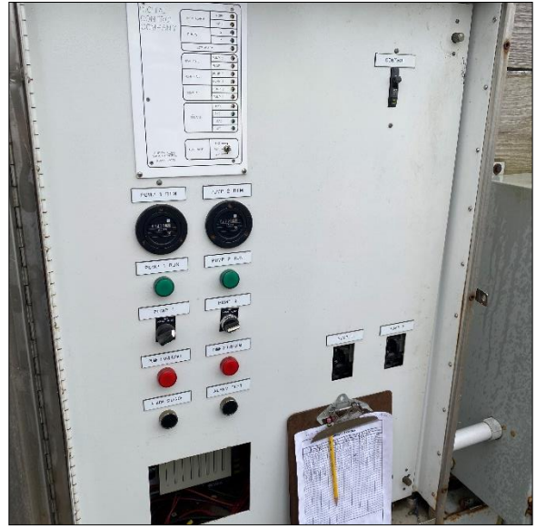
Figure 4 – Highway Lift Station Control Panel
