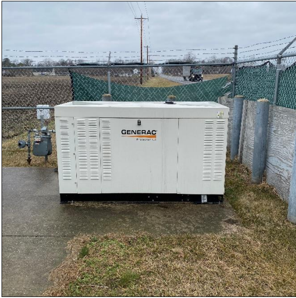
Figure 3 - Highway Lift Station Generator
