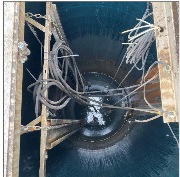
Figure 6 – Swan Song Grinder Station Wet Well
