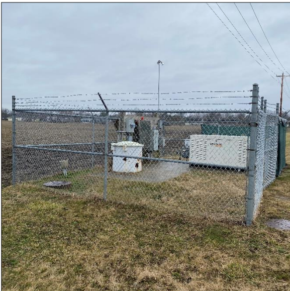
Figure 1 - Highway Lift Station
